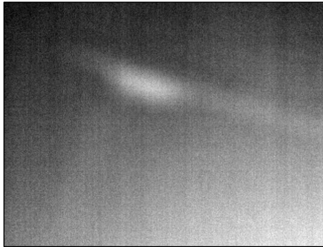
Figure 41: Hot Spot 2 on 4/28/12 at 1:00 PM (North Side of Wall 2)
