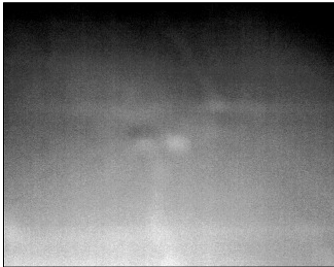
Figure A10: Thermal Image at Location 3 at 10:43 AM (North Side of Wall 2)
