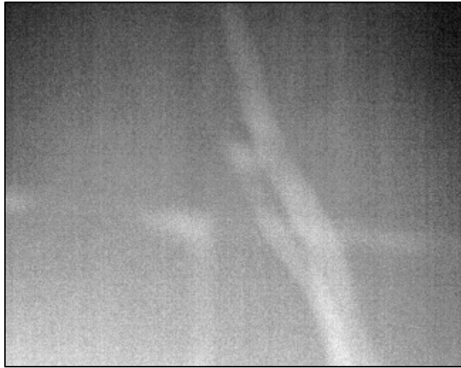
Figure A31: Thermal Image at Location 10 at 10:34 AM (North Side of Wall 2)
