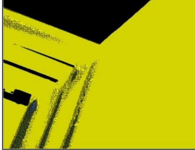
Figure 28: Color Thermal Image of Wall 2
